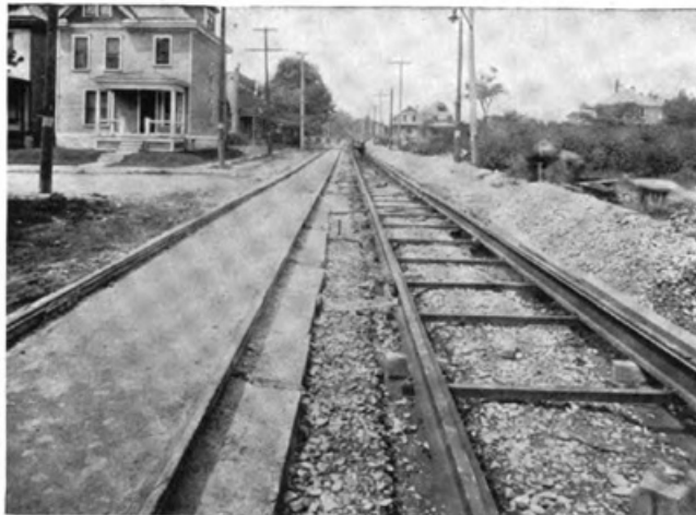
CONCRETE GIRDER CONSTRUCTION IN COLUMBUS. TO BE PAVED WITH BRICK. ONE TRACK CONCRETED. MATERIAL BEING DELIVERED IN OTHER TRACK
