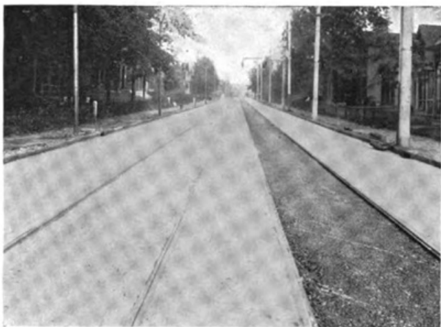
CONCRETE GIRDER CONSTRUCTION IN COLUMBUS. ASPHALT PAVEMENT COMPLETED, EXCEPT TOP COAT IN ONE TRACK
